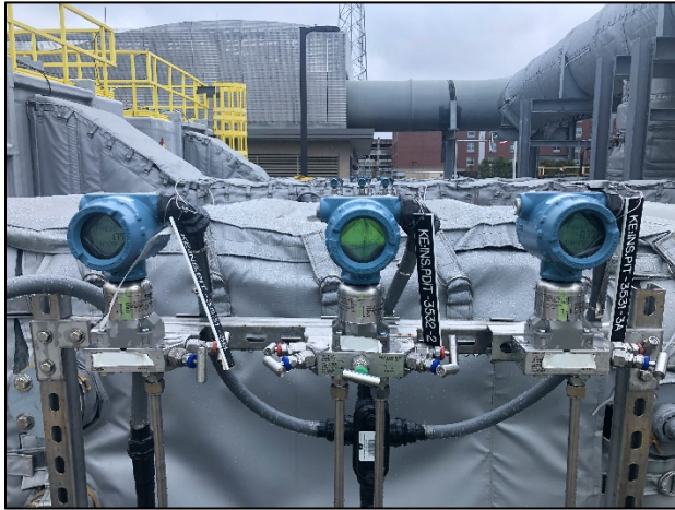
Odor Control Fan Pressure Transmitters
