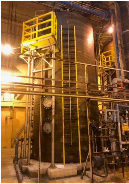
West Odor Control Wet Scrubber
