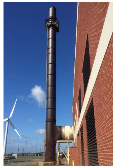
West Odor Control Exhaust Stack
