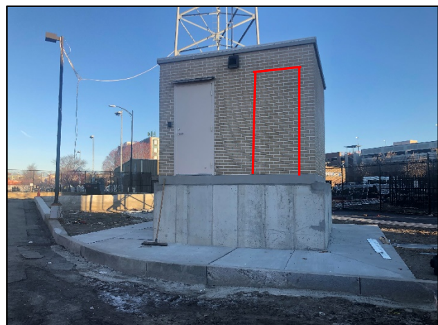
Communication Shelter Door Location (Actual)
